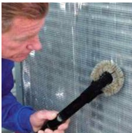
Evaporator coil is cleaned.
