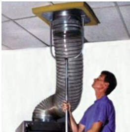
Negative Air Flow Unit Connected to System.
