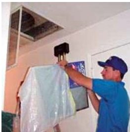
Return Air Duct is blocked.
